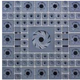
A Single Panel on the South Façade of the Arab World Institute
